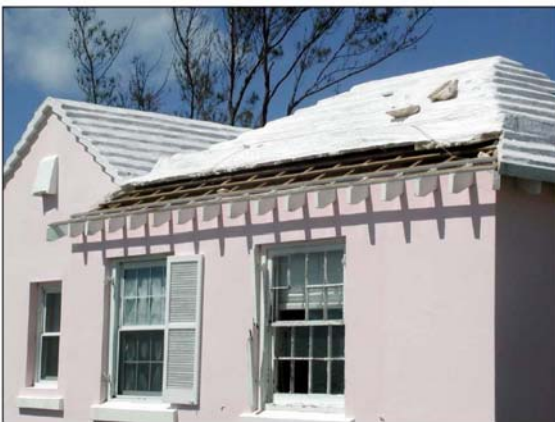
Figure 3. Typical leading-edge damage. Berry Hill Road, Devonshire (south facing).
