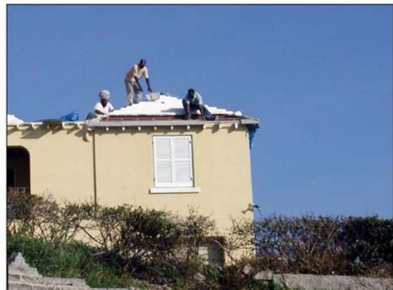
Figure 8. Leading-edge damage, Sayle Road, Smith's Parish (south facing).
