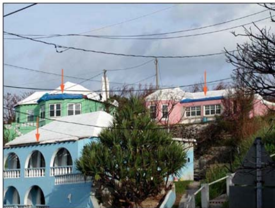
Figure 2. Widespread "leading edge" roof damage on south facing Mullet Bay Road, St George's.
