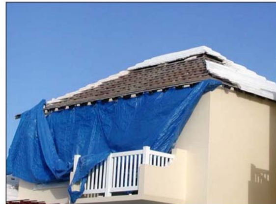
Figure 4. Less typical, extensive slate loss on windward side, St George's Club (south facing).
