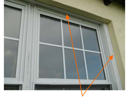
Windows with no visible caulking
