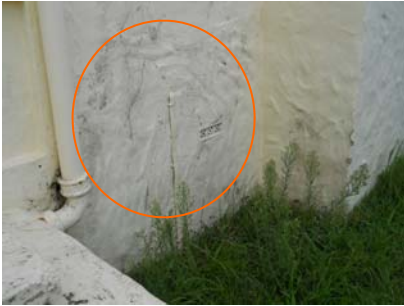
Hairline cracks, mildew and efflorescence
