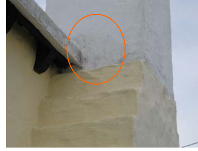
Hairline masonry cracks
