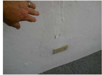
Flaking from recent repair
