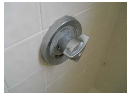
Tub/shower faucet looks pitted and aged.
