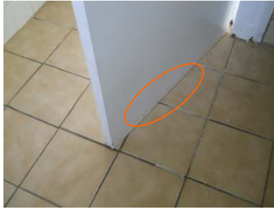
Door binds in bathroom. Shave.
