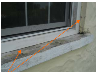
Caulking is missing
