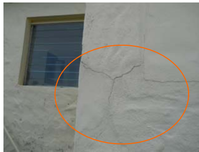
Masonry plaster cracks
