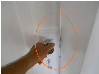
South bedroom door latch needs adjustment
