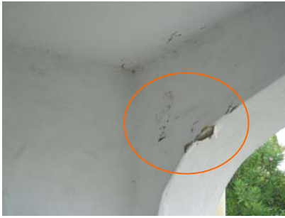
Efflorescence and flaking on north porch arches
