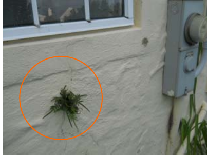
Plant growth in masonry walls indicates deferred maintenance
