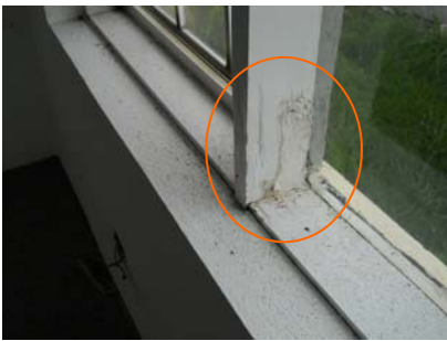
Wood frame rot in west picture window.
