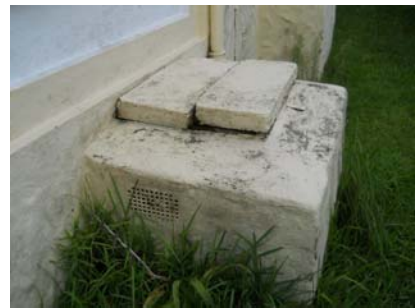
Tank access slabs should be replaced with galvanized frame & lid with locking bar.
