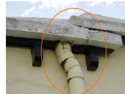
Mold indicates long term moisture issue with cracking and seal around downpipe
