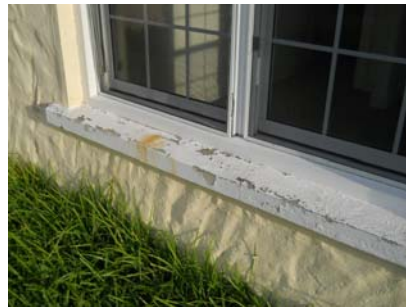
Flaking paint on window sill
