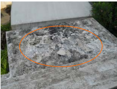
Significant spalling on flat roof, west side.
