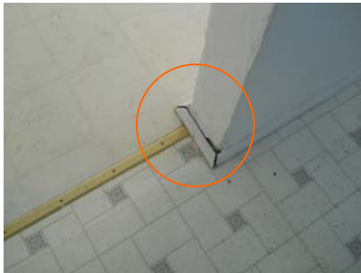
Kitchen to laundry room transition. Base trim requires repair.
