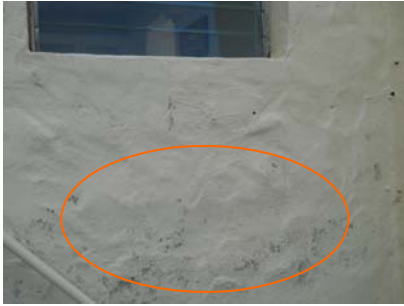
Mildew from excessive moisture in stone.
