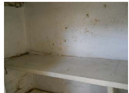
Efflorescence and degradation inside laundry room cabinets
