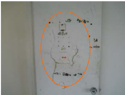
Interior bedroom door requires replacement.
