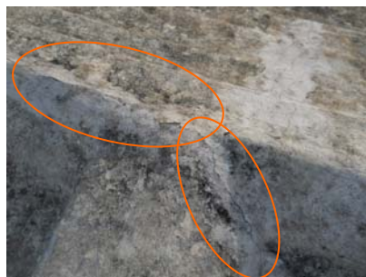
Roof cracking. Repair
