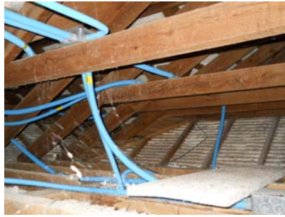
Blue flex conduit indicates relatively recent rewiring.
