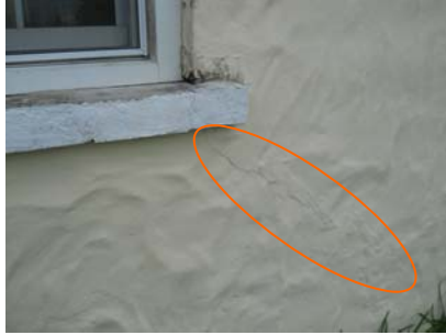
Masonry crack. Previous repair noted.
