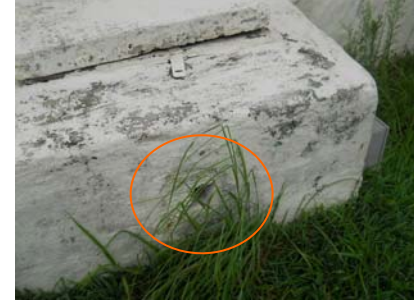
Tank overflow. Replace wire mesh screen
