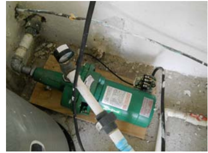
Water pump is relatively new and functional
