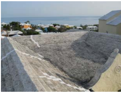
Recent repairs shown bright white. Significant discoloration indicates deferred maintenance.
