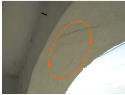
Minor cracking possibly from corroded rebar. Monitor
